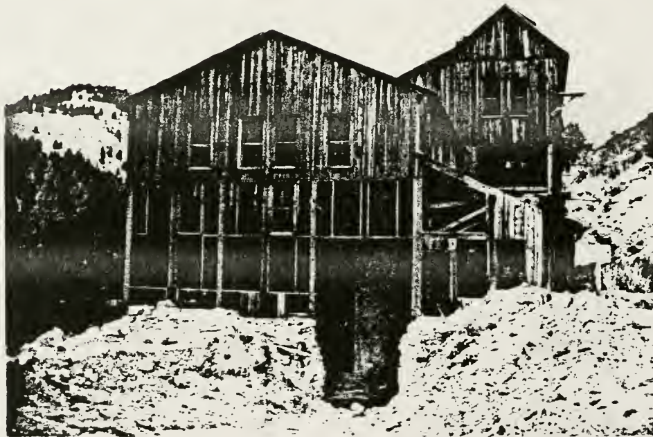
Figure 153. Arsenic plant (structure #59) showing opening in stone foundation made for equipment entrance during clean-up of hazardous wastes, north view.
